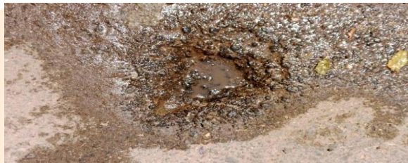
Fig.9. Pothole Present in our Campus.
