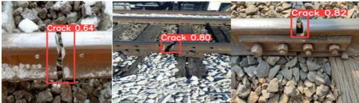
Fig: output of crack detection
