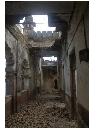
Figure 3 Collapsed roof and damaged flooring in the corridor.
