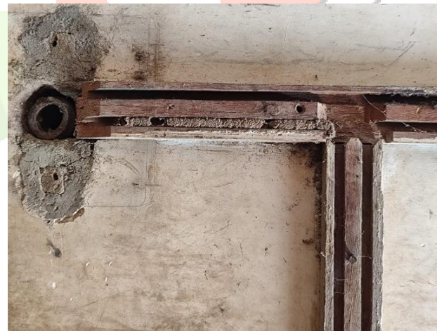
Figure 4 Old electrical wooden lines
