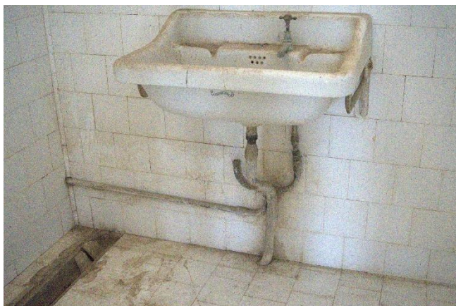
Figure 5 Old plumbing connection
