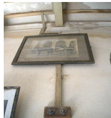
Figure 6 Old electrical switch board
