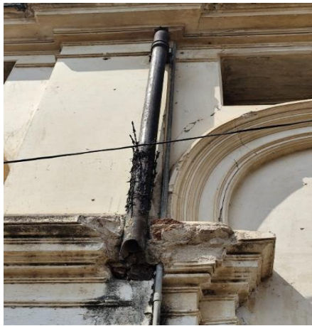
Figure 3 Broken Plumbing pipe
