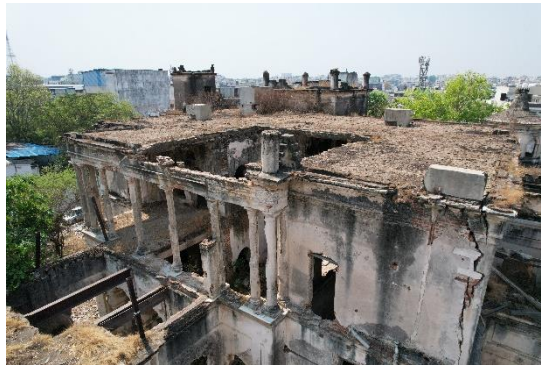
Fig. 11: Broken terrace floor in first floor
