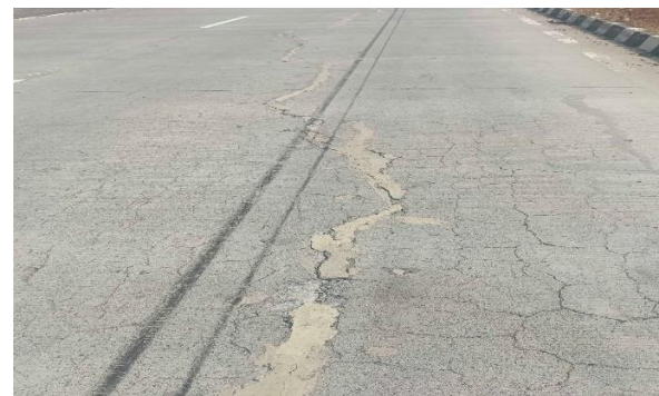
Fig. 2. Wear and tear of the polymer base epoxy sealent and cementious grouting
