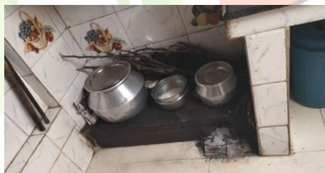
5.3.1 Inbuilt Metal Stove
