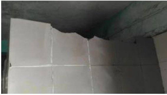
Fig.1 Broken Dado of toilet block
