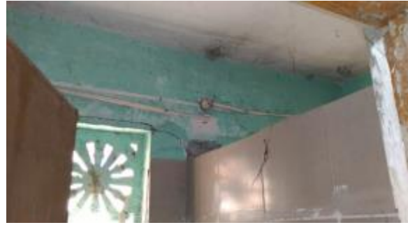
Fig.2 Damaged electric system
