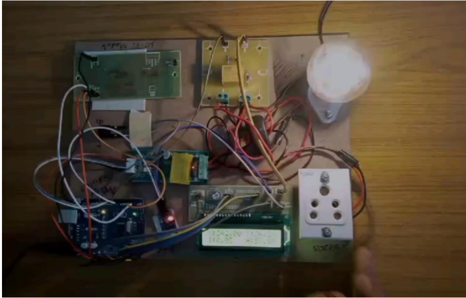
Figure 5 Kit to monitor and control single phase system using IoT
