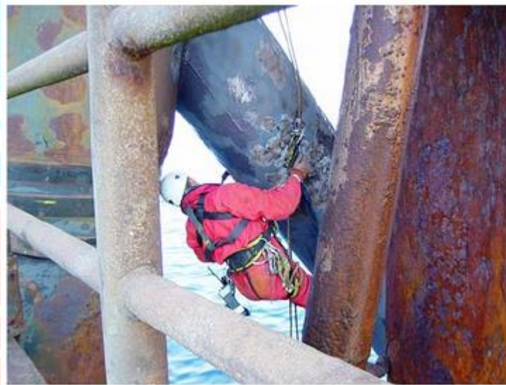
Figure 1: Corrosion of steel on offshore structure due to premature failure of coating. Courtesy of Hempel A/S
