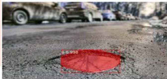
Fig -3: Detected Pothole
