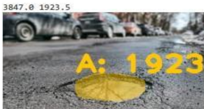
Fig -4: Detected Pothole with area
