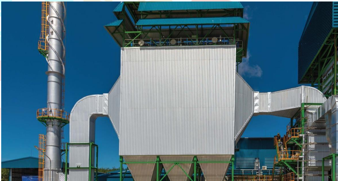
Figure 1.2.1. ESP Used in Power Plant
