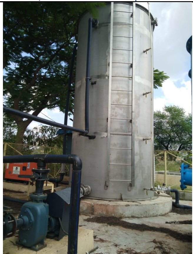
Photo 3: 25 KLD STP based on granular sludge process (courtesy M/s Shreyans Energy P Ltd)
