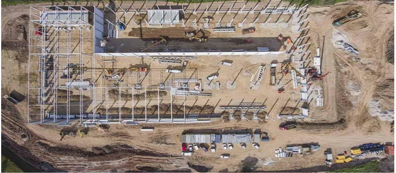
Figure 1 Aerial image of construction site in Pune Maharashtra taking by (matrice 300 rtk) drone.
