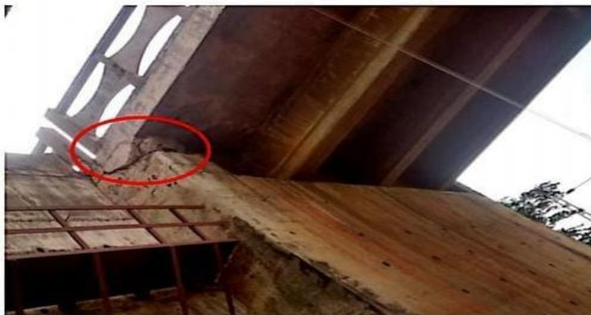
Distressed earthquake arrester
