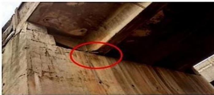
Concrete spalling, reinforcement exposed at ends of girder
