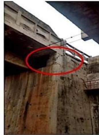
Distressed earthquake arrester
