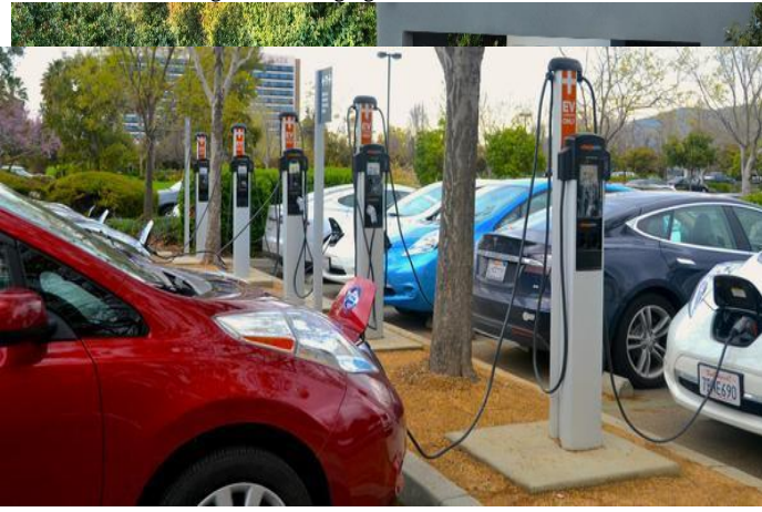
Fig 3. EV Charging at Home Station
