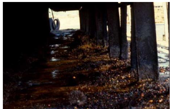
Figure 4 Palm oil FFB receiving bay
