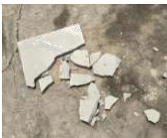
Fig 7. CB cracks & detachment
