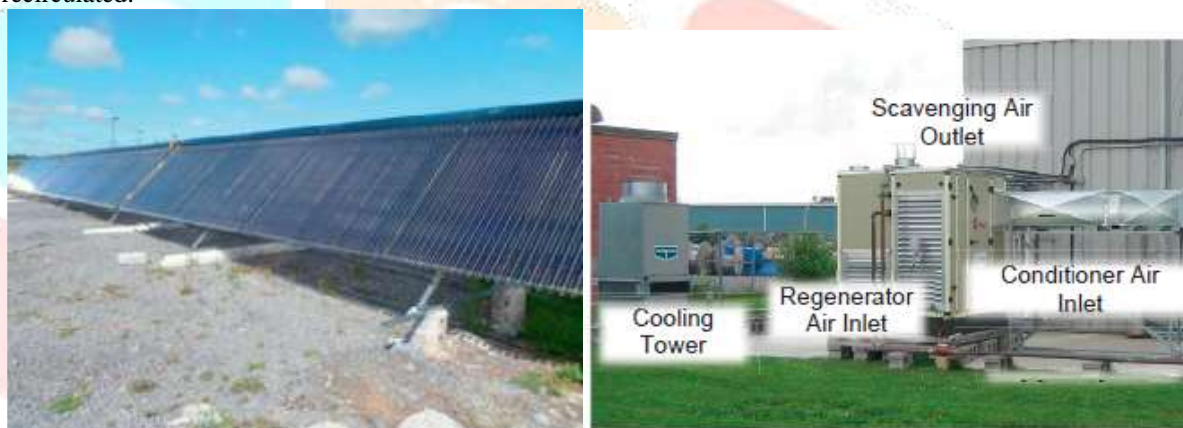
Fig 2. (a) Installation of solar array (b) Liquid desiccant air conditioner (right) at field testing site [5]
