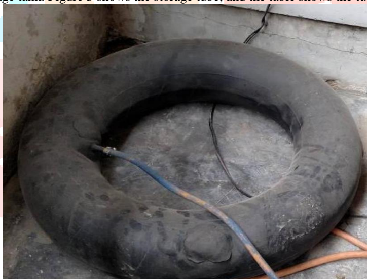
Figure 3 : Biogas storage tube
