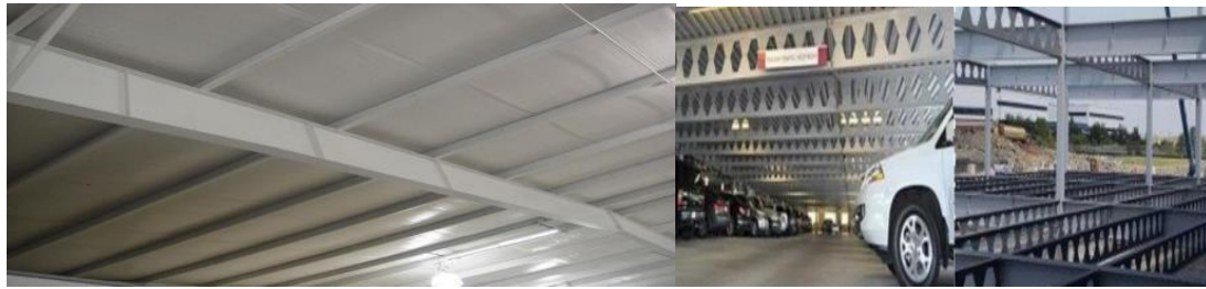
Fig 1.1: Roof Structure (a) (b) Fig 1.2: (a) Parking Roof Castellated Beam Structure, (b) Cable Carriage Racks
