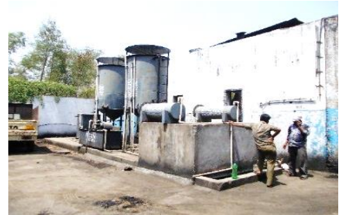
Photograph-3: ETP at Jaika Motors, Nagpur
