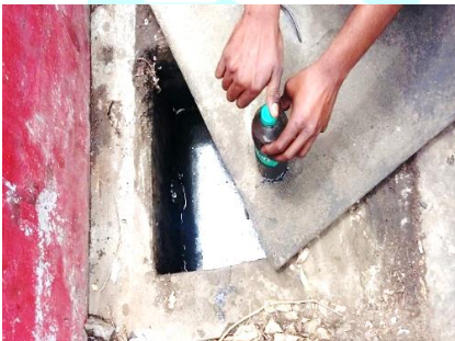
Photograph-4: Wastewater collection tank of Service Station at Swawlambi nagar, Nagpur
