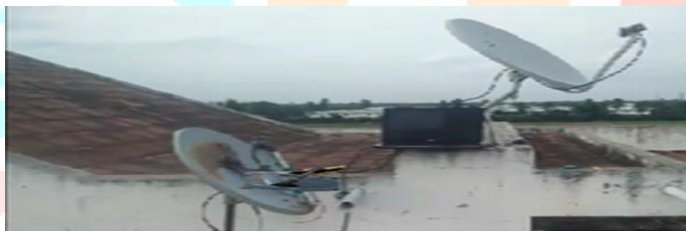
Figure 19. Design of SAT FMDH Antenna for Improve Internet speed.
