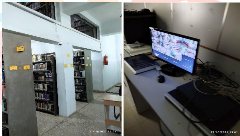
Fig .3 CCTV Surveillance, between the Racks cameras installed, video backup monitoring screen at librarian desk and fire safety equipments in the Engineering college library
