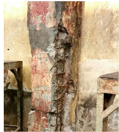
Corrosion of Rebar
