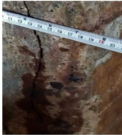
Wider cracks on Column
