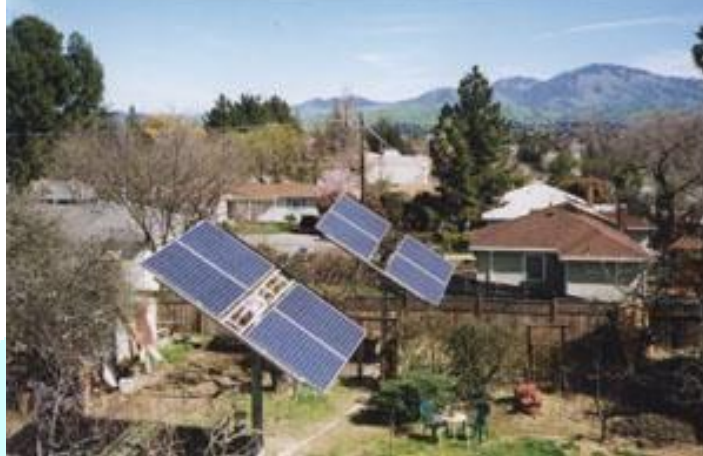
Fig. 2.1. Backyard installation of passive single-axis trackers, rated at 2340 watts.
