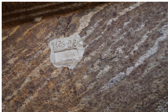
Figure 4 Measuring Developing Crack by Cement TALE TELL
