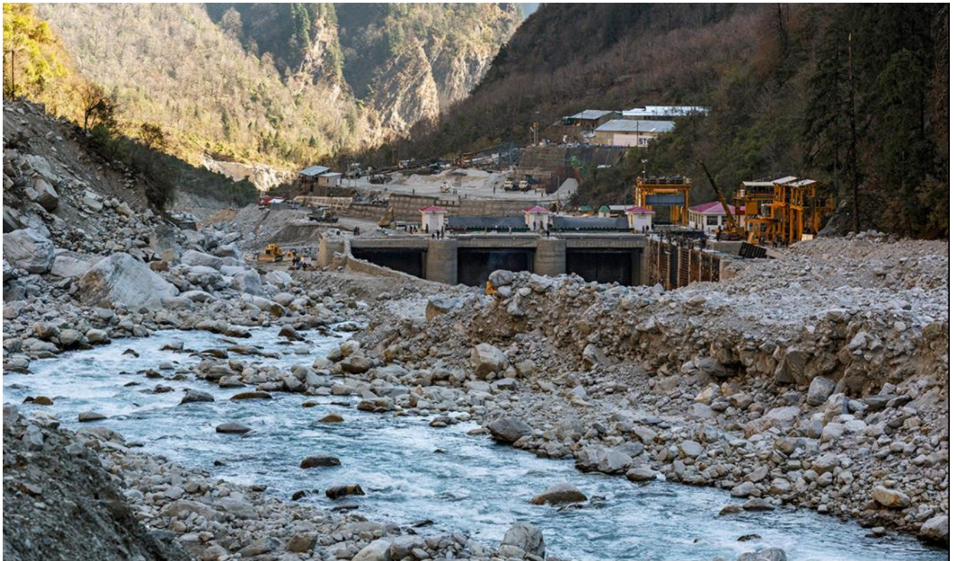
Fig 10. Vishnuprayag Hydroelectric Project on the Alaknanda River damaged by the flashfloods
