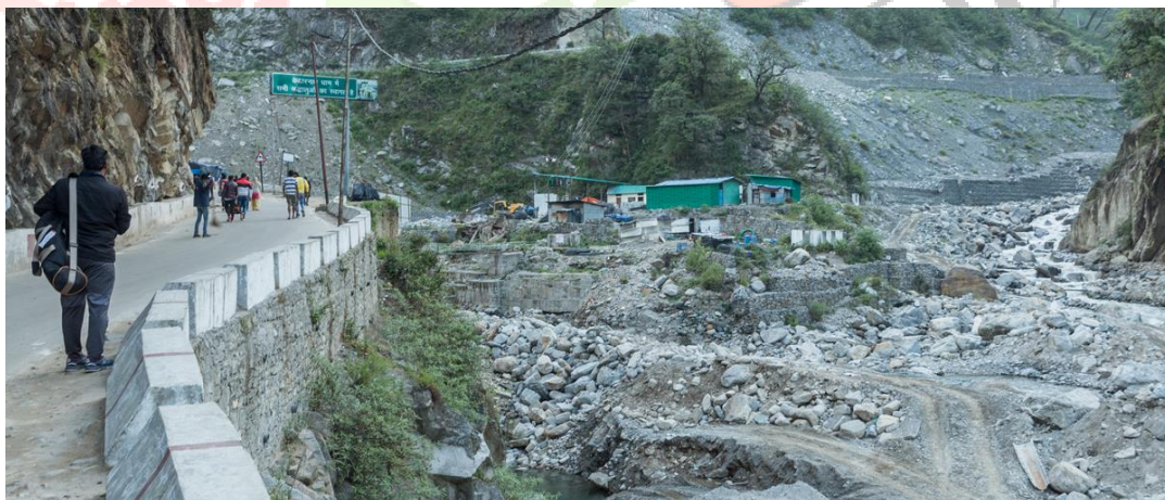
Fig 9. Construction debris and activities along Mandakini River near the base from where the trek to Kedarnath begins
