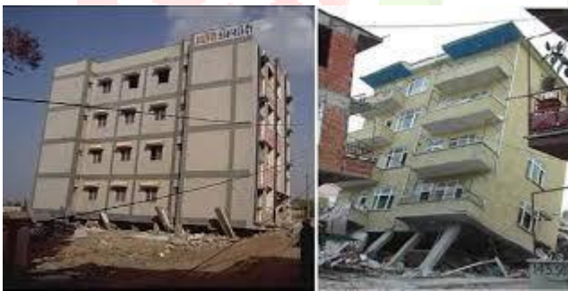
Figure 4.1. Failure due to large lateral displacement in soft storey
