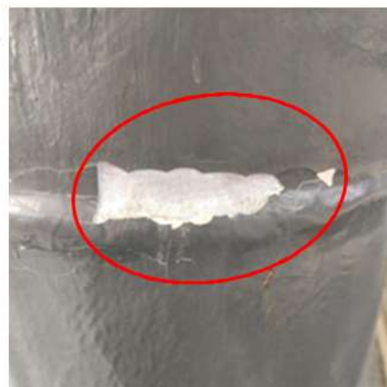
Figure 5 Top coat peeling off
