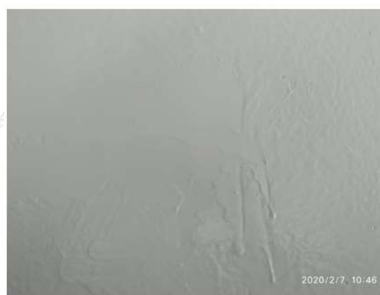
Figure 3 Sagging of paint due to inappropriate mixing of coatings
