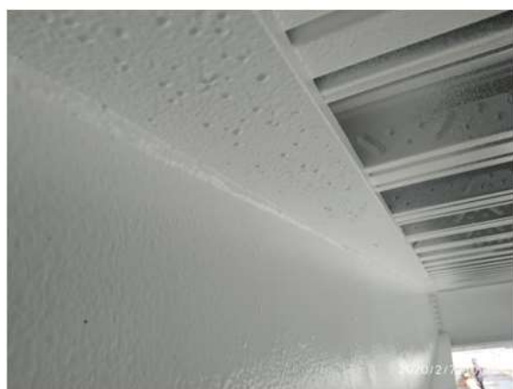
Figure 2 Bubbles formation in thin film Intumescent coating
