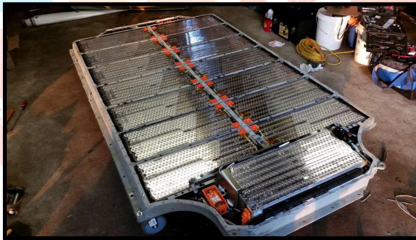
Fig 1: Lithium-ion Battery pack [15]
