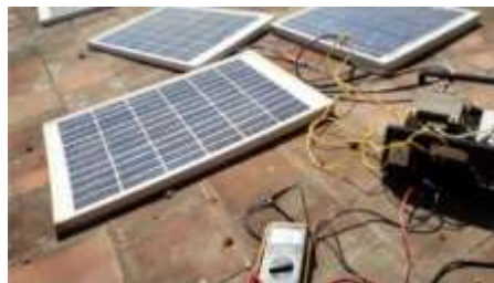
Fig.8 Test Case: Testing Solar Panel and UPS without Load
