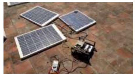
Fig.9 Test Case: Testing Solar Panel and UPS Connection
