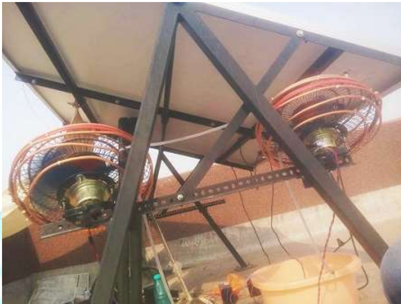
Fig 2 Air cooling system of solar PV installed at roof of building UTD RGPV Bhopal
