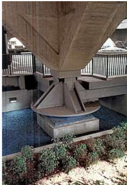
Close-up of abutment of seismically retrofitted Municipal Services Building in Glendale, California
