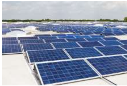
Fig no.1: Solar panel
