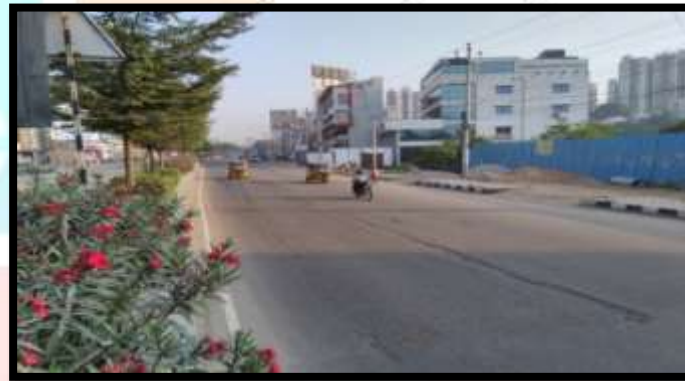
Fig1.2 Formation of Longitudinal Cracking
