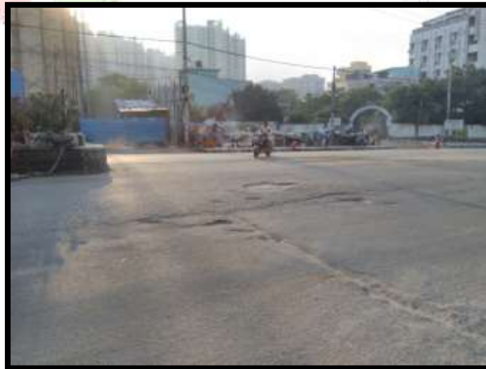
Fig 1.3 Formation of Transverse Cracking
