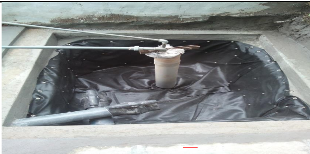
RWH PIT with Geo fabric membrane.
