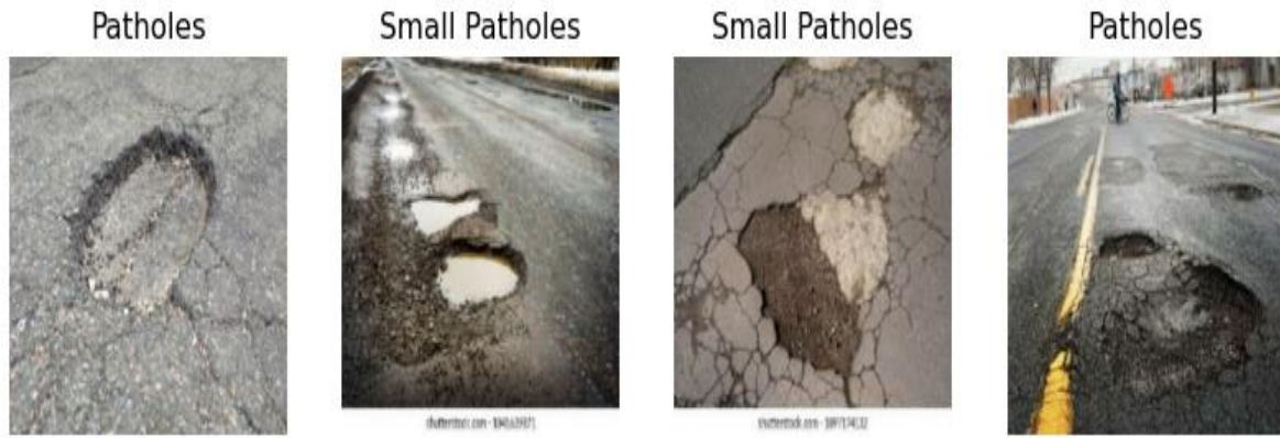
Figure 1: Pothole input images
