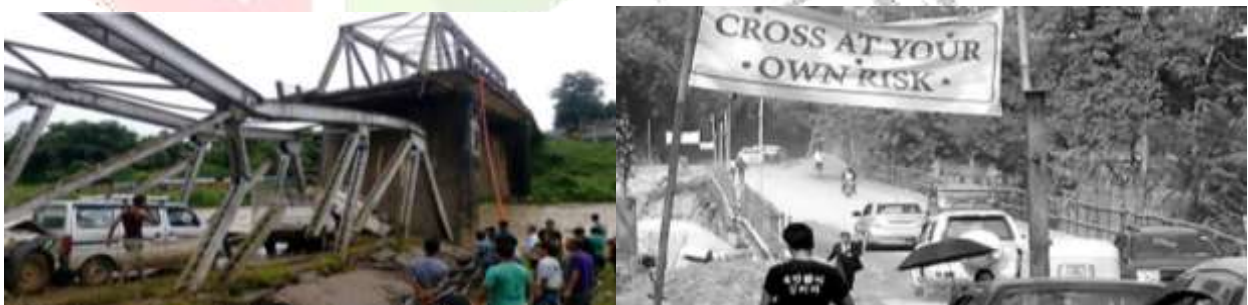
Fig.1.2. Collapse of Dhansiri Bridge, Nagaland.
