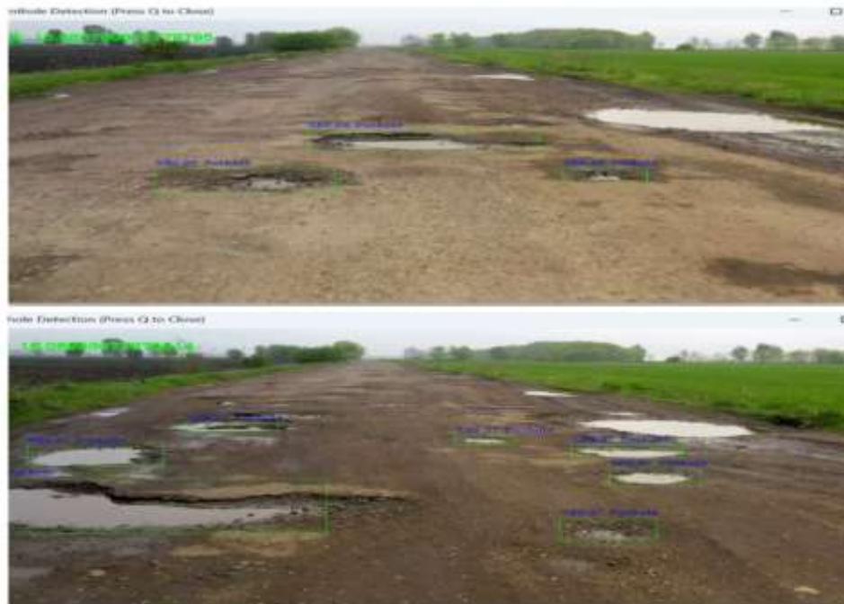
Figure 6 . Potholes on Roads
