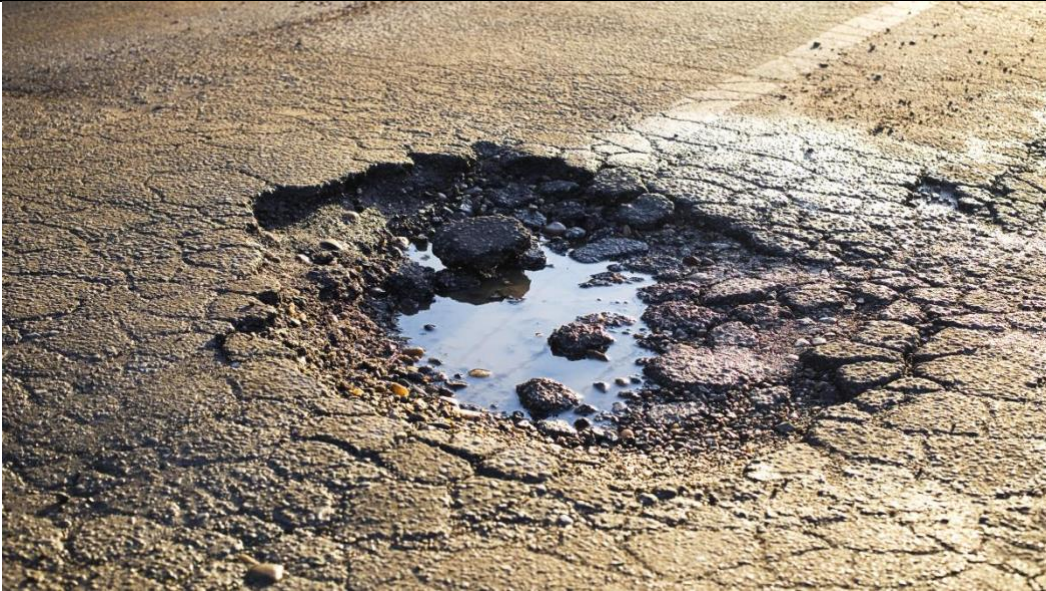
Bituminous road potholes
