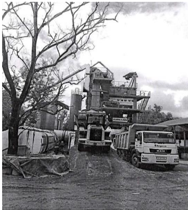
Fig. No.03: Hot-Mix Plant (Ammann Appollo, 180 TPH)
