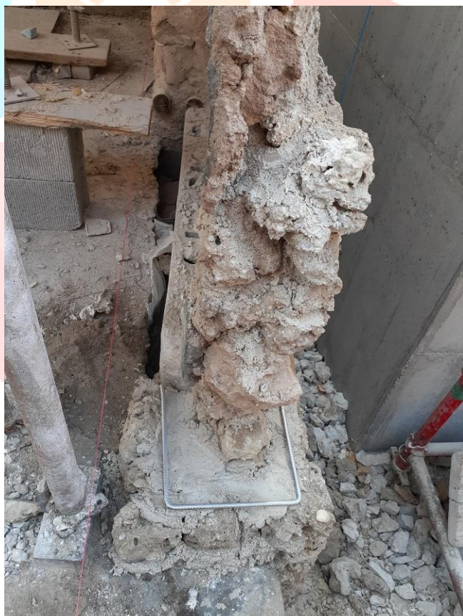
Fig.1. Damaged wall before conservation
