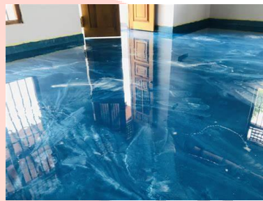
Fig4. epoxy used in flooring
