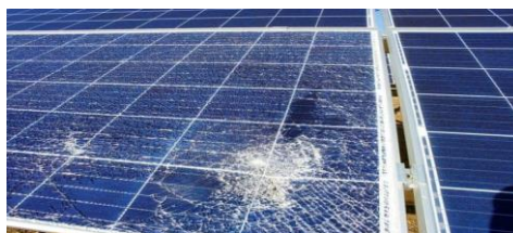
Figure 5: the presence of broken glass on solar panels increases their susceptibility to potential weather-related damages in the future.
