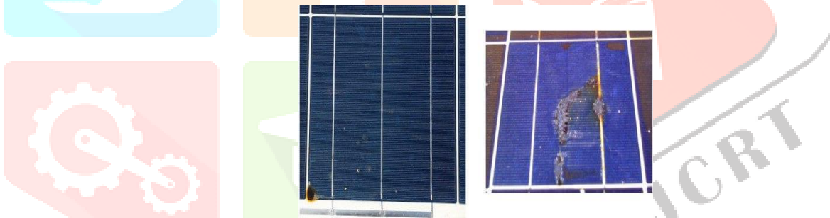
Figure 2: the occurrence of hotspots due to faulty solar cells has the potential to trigger a fire hazard
