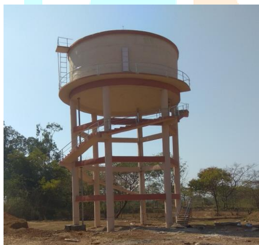
Figure 3.2: Water Tank to supply water
