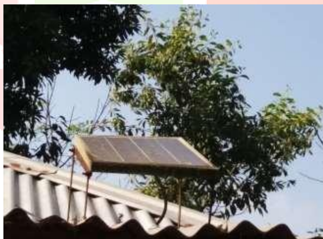
Figure 3: Pico-Solar Panel Set Up on the House Roof
