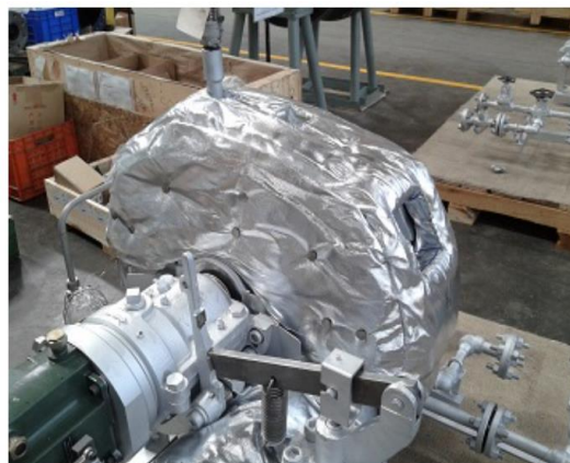
Figure: 10 Glass wool gearbox insulation
