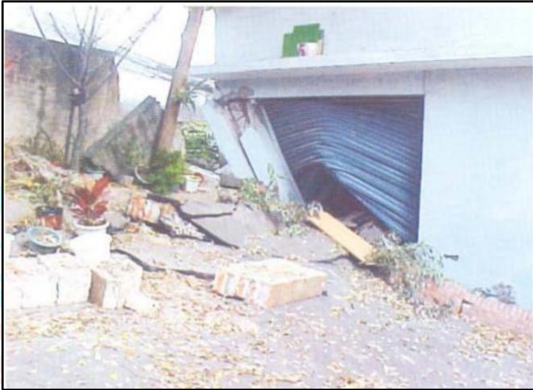
Fig.1 Damage of building due to ground failure
