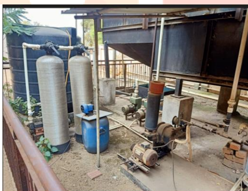
Photo 1 – EC reactor used as domestic waste water recycler
